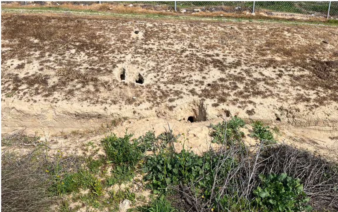
Figure 10. Photograph of the wastewater treatment plant, looking north, showing a storage pond bank with signs of herbicide use and ground squirrel burrows.
