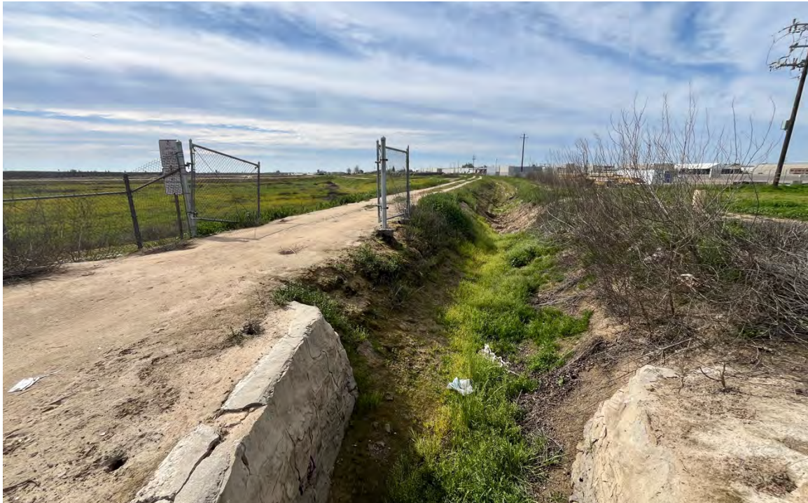
Figure 12. Photograph showing Garfield Ditch along the western boundary of the wastewater treatment plant portion of the Project site, looking southwest.
