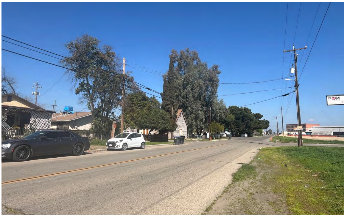
Figure 6. Photograph of a sewer line work area, looking north along South Del Rey Avenue, showing ornamental trees and residential and commercial development.
