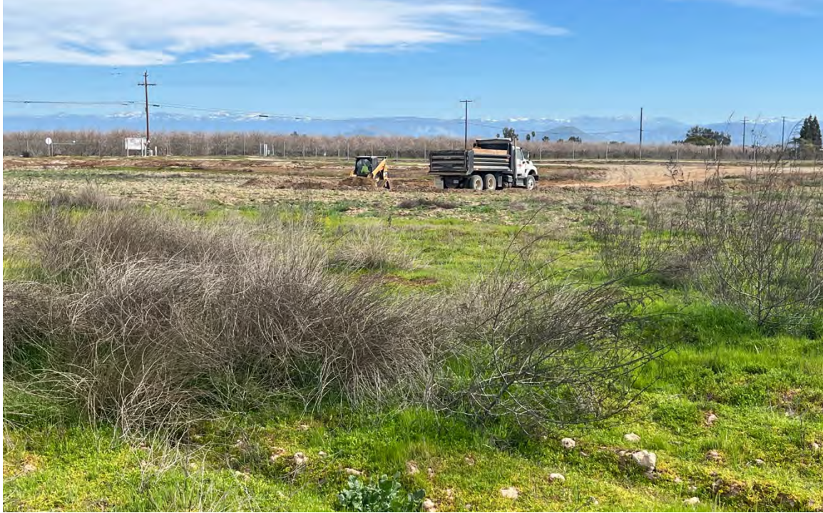
Figure 11. Photograph of the wastewater treatment plant, looking northeast, showing construction in the north pond basin of the wastewater treatment plant.
